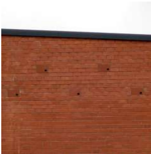
Antrim Public Library, Northern Ireland: Ibstock Swift bricks were used to bring life to this featureless wall
