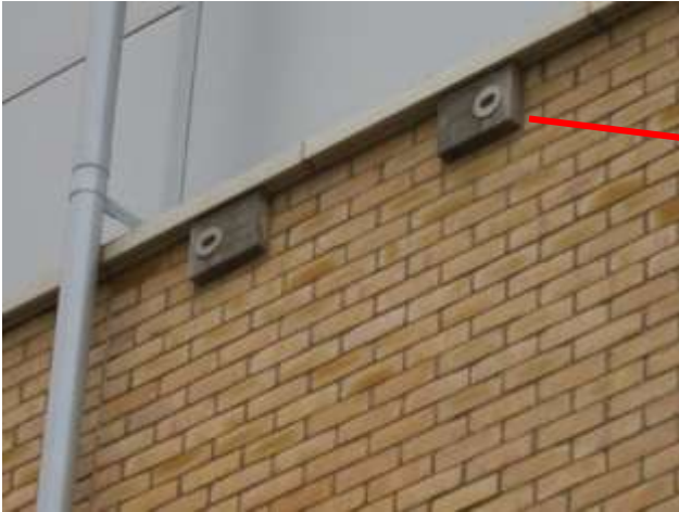
Two Schwegler Swift Bricks installed in the walls of the Maternity Unit at the Lister Hospital
