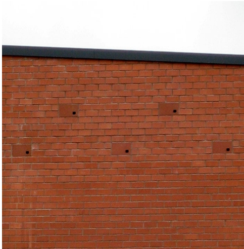
Antrim Public Library, Northern Ireland: Istock Swift bricks were used to bring life to this featureless wall
