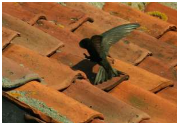
A Swift entering a roof via a displaced pantile. The nest is on the roofing felt below Photo © Bill Ball
